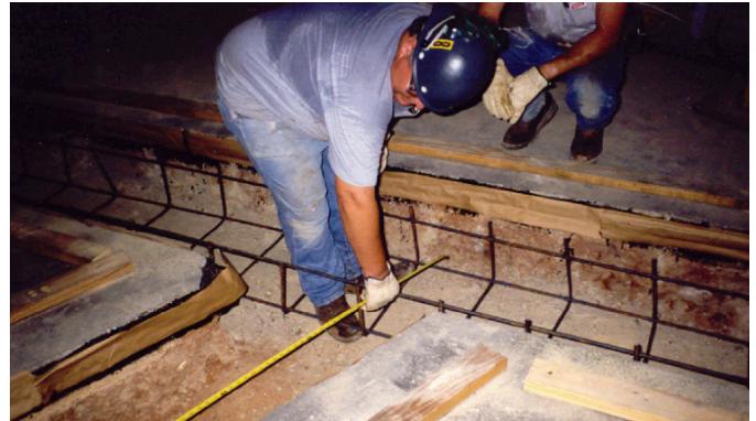
3. New trenches were saw-cut into the existing concrete floor. The customer elected to excavate a space large enough for the trench liners, plus 6 inches of clearance for new reinforcing steel. An expansive water stop was used on the saw-cut face of the existing concrete.
