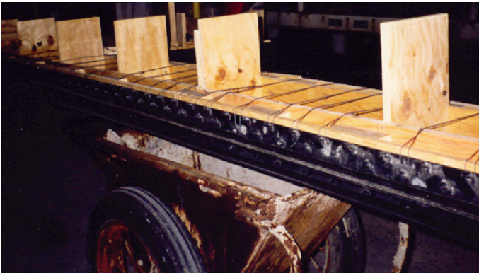
2. Closely spaced tie wires secure the forms inside the liner to prevent deformation of the trench liner bottom during concrete casting. Wires are tied to the top row of anchors. No penetrations are made in the liners to attach the formwork. Without this restraint, the forms could be pushed out of the liner, creating a bulge in the bottom of the trench.
