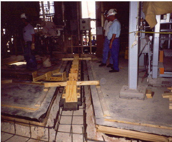
6. The trench liners are hung in the excavation by the 2 x 4 cross beams to ensure adequate clearance between the liner and reinforcing steel and to set the invert elevations.
