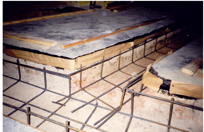
4. Note the 2 x 4s along the sides of the trenches. These are used to support the 2 x 4 cross beams from which the trench liners are hung.
